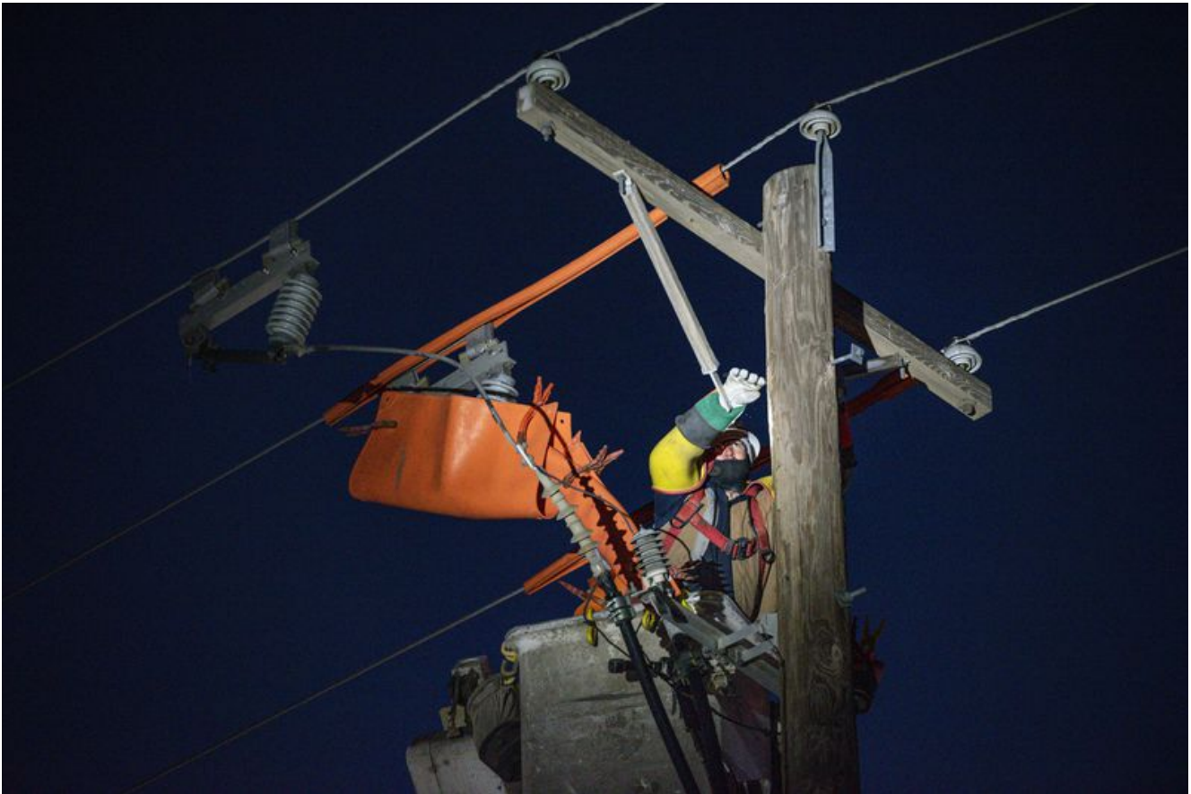
Oncor apprentice lineman Brendan Waldon repairs a utility pole that was damaged by the winter storm that passed through Texas Thursday, Feb. 18, 2021, in Odessa, Texas. (Eli Hartman/AP)
