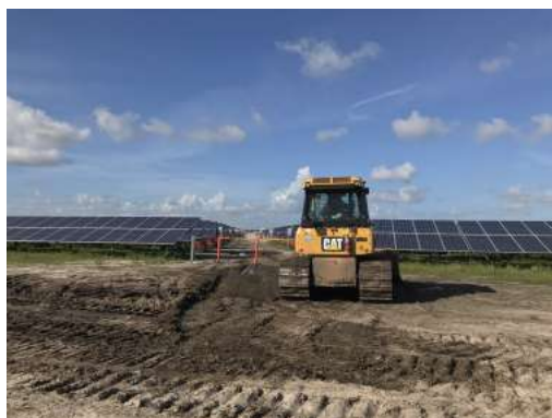
A worker prepares the ground at Florida Power & Light’s Indian River solar-energy center, under construction near Vero Beach, Florida. Jamie Smith Hopkins / The Center for Public Integrity
