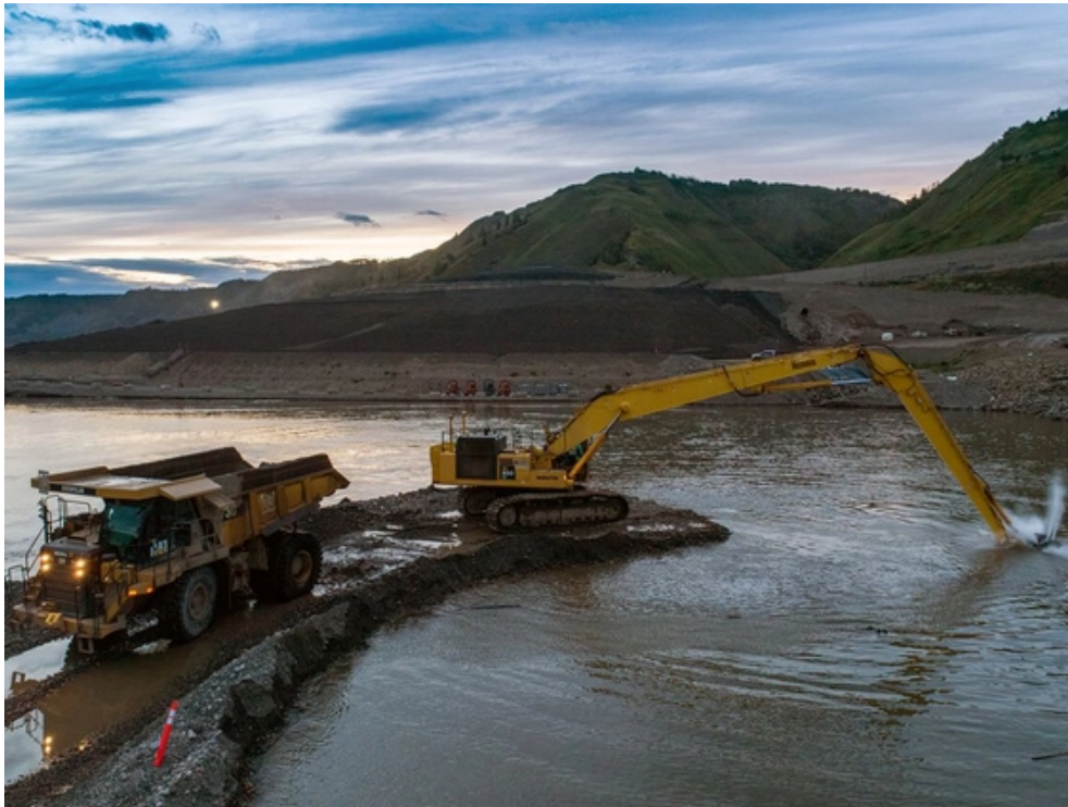
An excavator dredges out a channel at the entrance to one of the river diversion tunnels on B.C. Hydro's Site C dam project on the Peace River near Fort St. John in August. PHOTO BY B.C. HYDRO.
