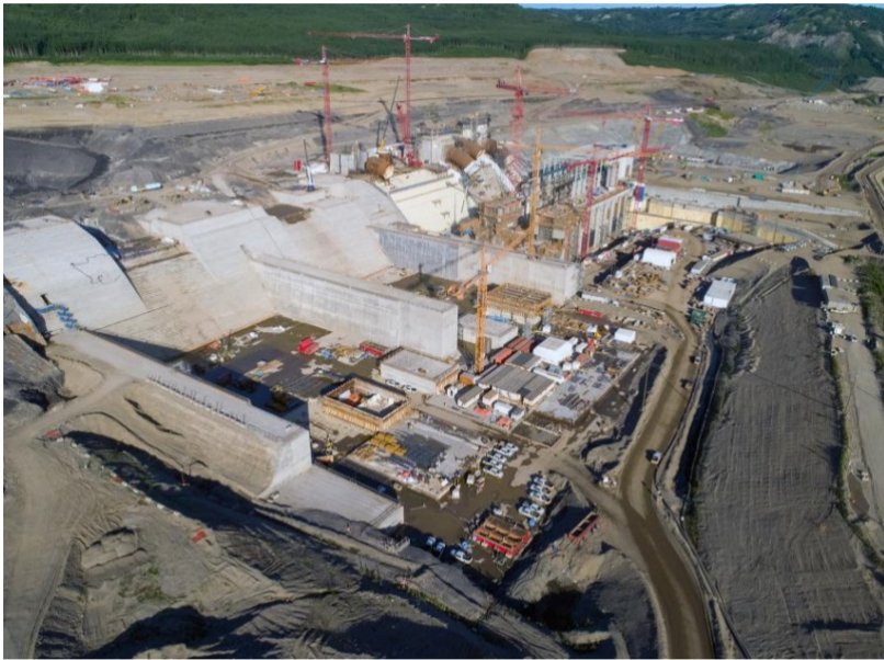
Aerial view of the Site C spillway headworks, stilling basin, intakes, penstocks, and powerhouse, June 2020. Photo By BC HYDRO
