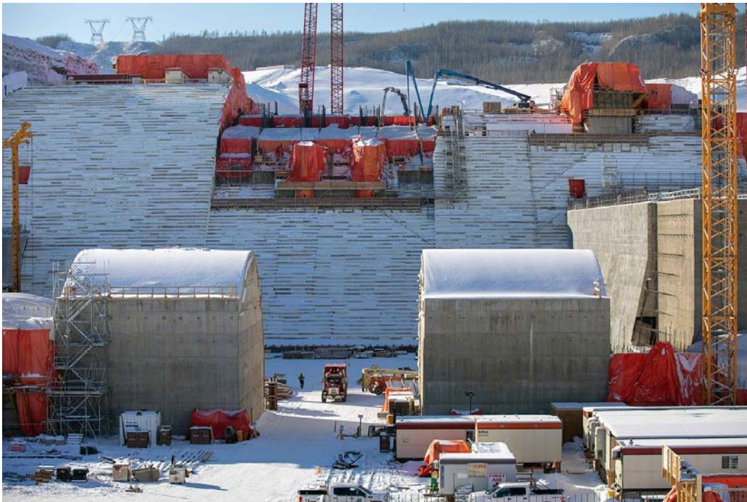
Crews pour concrete at the Site C dam construction site in February, 2021. Photo: BC Hydro
