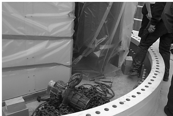
Figure 8: The switchgear and transformer on top of the concrete foundation ready for placement of the tower.
