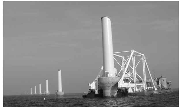
Figure 7: The floating crane with a foundation and the lower part of the tower at the site just before installation.
