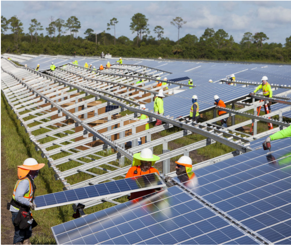
Workers install panels last year at the Babcock Solar Energy project in Punta Gorda, Florida. The project is one of eight new utility-scale solar farms in the state set to be completed by early 2018. FLORIDA POWER & LIGHT
