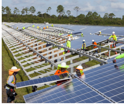
Workers install panels last year at the Babcock Solar Energy project in Punta Gorda, Florida. The project is one of eight new utility-scale solar farms in the state set to be completed by early 2018. [Photo courtesy Florida Power & Light]
